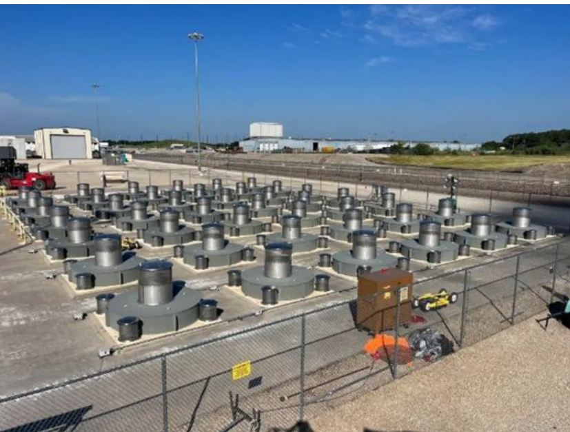
Future HOLTEC HI-STORM UMAX
