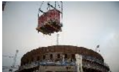
Modular pool construction accelerated on Unit 2. Improved method included changes to the supply chain and increased ability to manufacture components at Site – reducing schedule risk.
