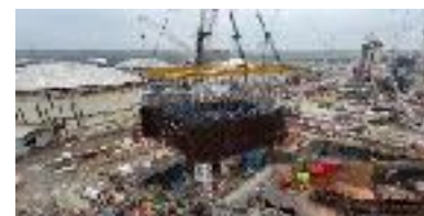
Staircase "mega lift" saved 70% of installation time and allowed concrete to be poured 9 weeks faster.
