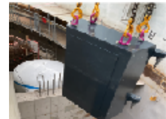
At the point of dome lift, 44 "nuclear" doors were installed in Unit 2 versus 28 on Unit 1. There was 30x the amount of steel fitted on U2 vs U1 at the point of dome lift.
