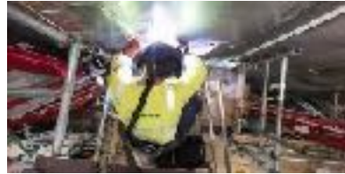
Welding of stainless-steel pools For Unit 2 a different welding technique has been used on large pools. On Unit 1 panels got too hot and work slowed. The new technique (SMAG) alleviates this.
