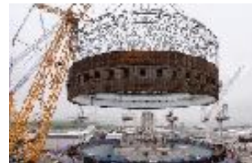
Liner ring 3 was installed two months ahead of schedule on Unit 2. The welding of the ring to the Unit 2 Dome was achieved 90 days faster than Unit 1.
