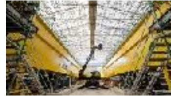
Unit 2 Polar Crane assembly Improved logistics and tracking of components, plus greater assembly at ground level is enabling Unit 2's Polar Crane to be built 30% quicker
